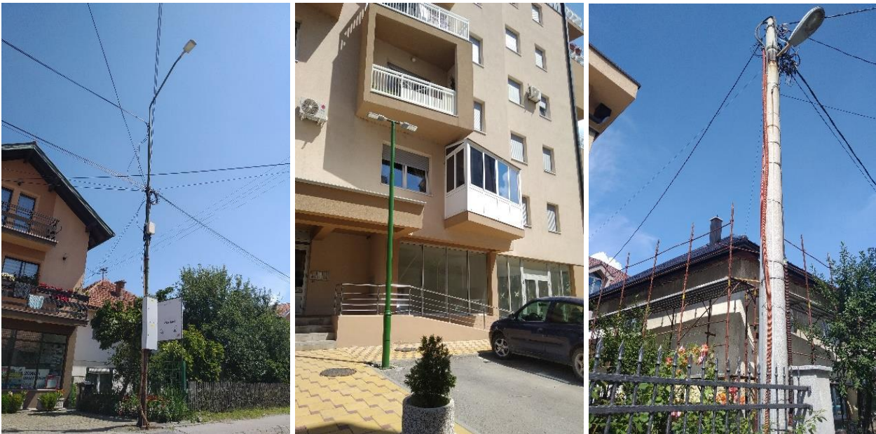
Image 29: Poles (unauthorized cabling - left, under ground cabling – centre, over ground cabling – right)
