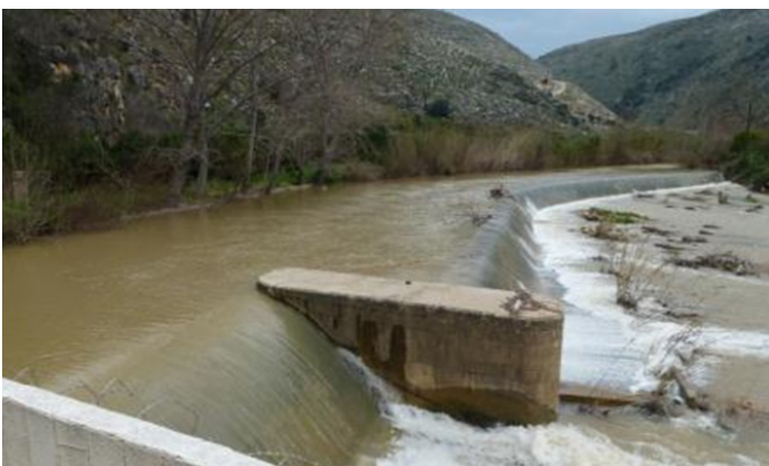
Figure 18 Qasimia irrigation intake
